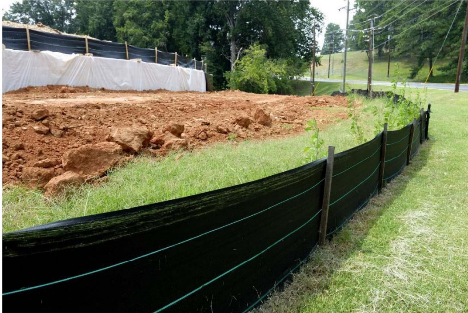
Figure 5.3 Example of Silt Fencing
